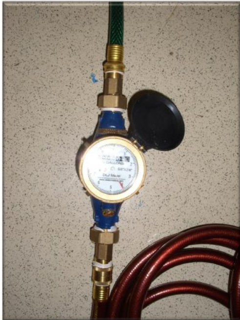
Figure 16: In-Line Flow Meter
